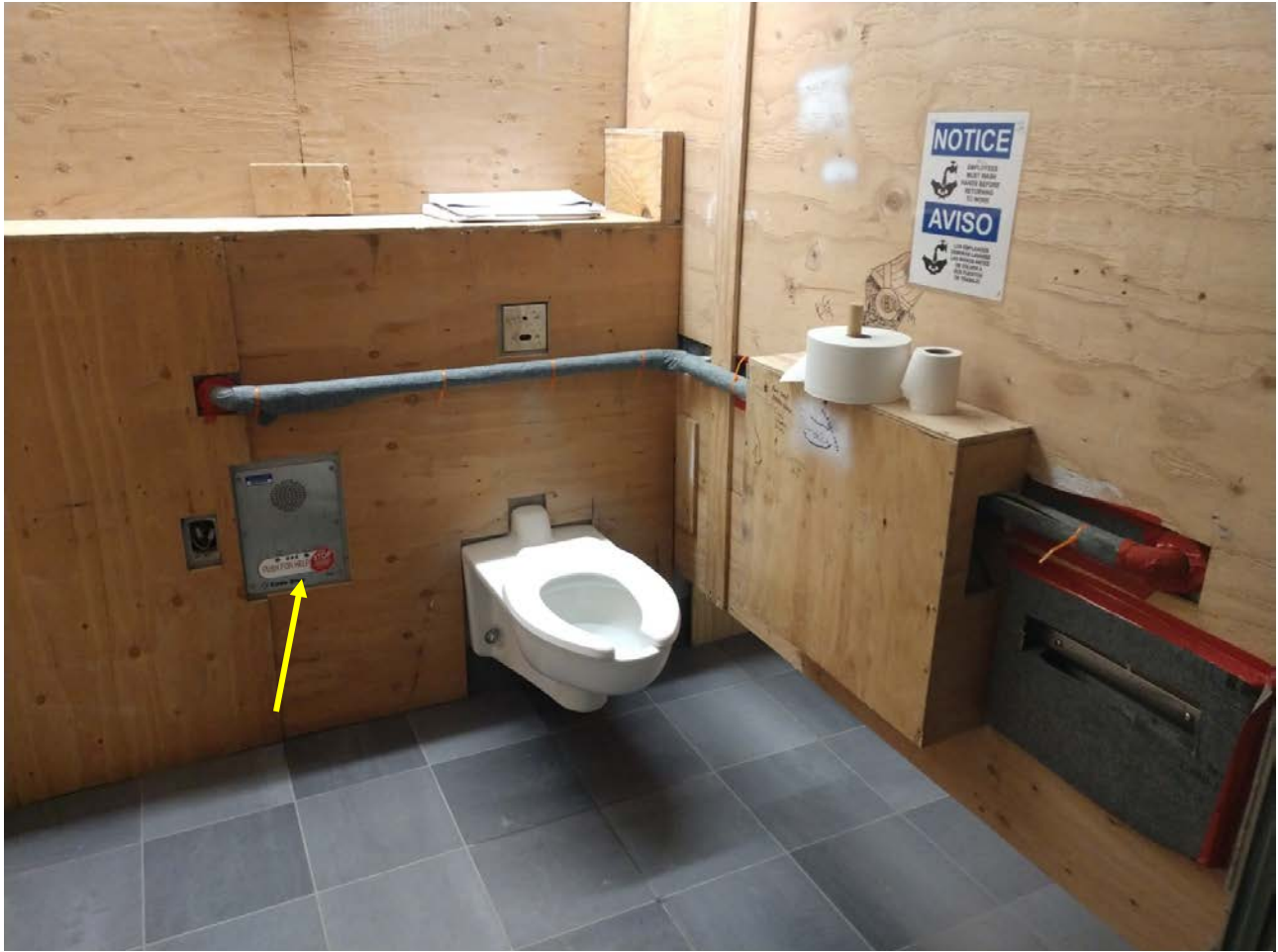
Pictured above is the accessible stall in one of the restrooms. The walls are covered by wood. A grab bar is visible above the toilet. To the left is a panic box with button for emergency calls if needed.
