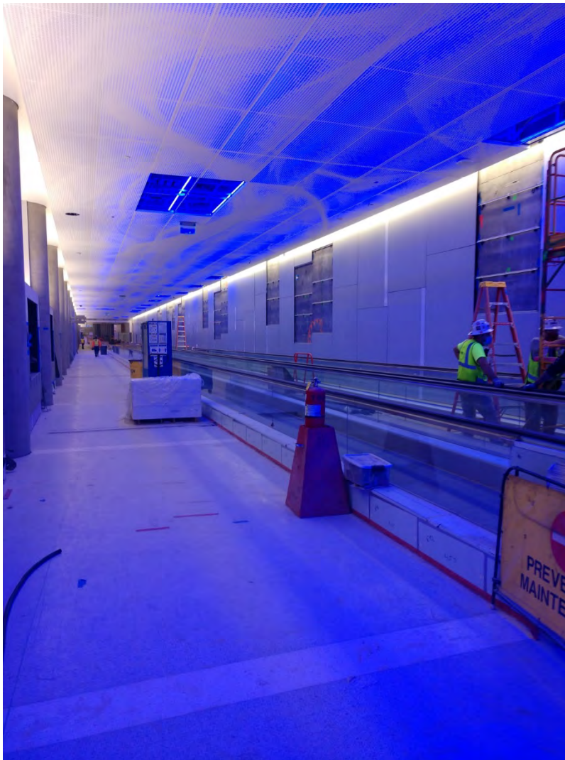
Pictured is a very long corridor, which is part of the Passenger Tunnel (PAX). To the right is a movable walk and to the left is a walkway for persons who want to walk the distance from Bradley West to the Midfield Concourse. On the wall to the right are panels where messaging and advertising will be located.
